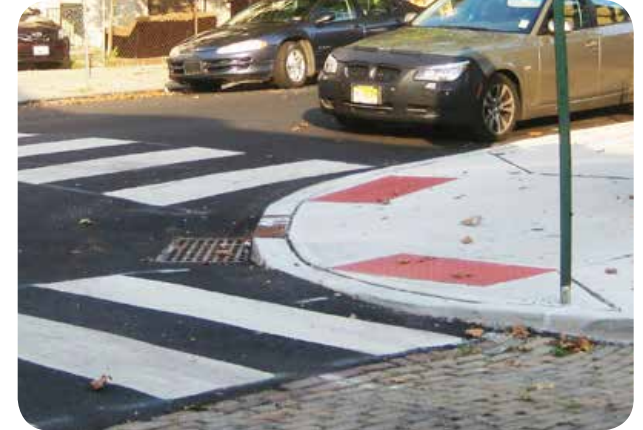
Intersections should have two perpendicular, ADA-compliant curb ramps per corner. Image: The RBA Group
