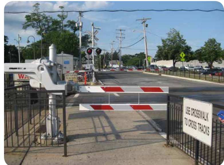
Pedestrian gate with “gate skirt” being tested at the Aberdeen-Matawan Train Station. Image: The RBA Group
